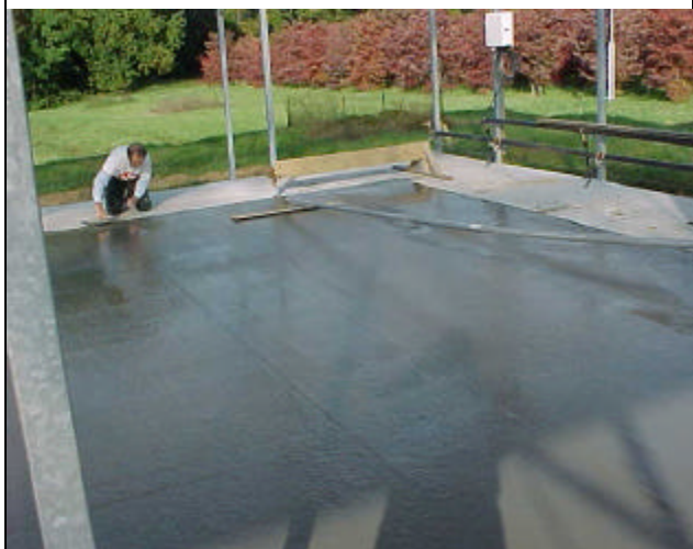
View showing the finished floor and CCEA Faculty member Dave Mears doing an edging procedure.
