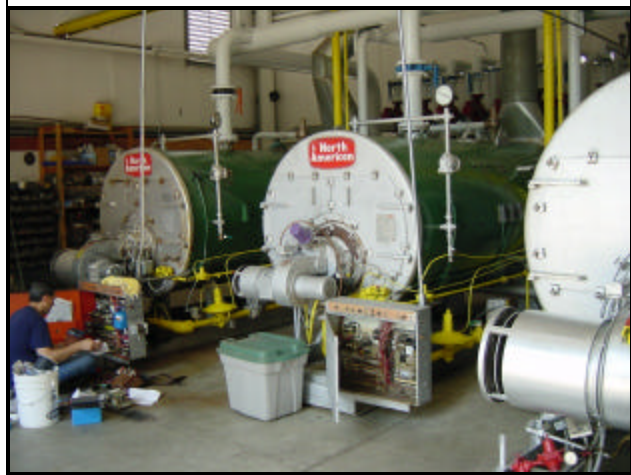
Use the summertime for boiler maintenance.
