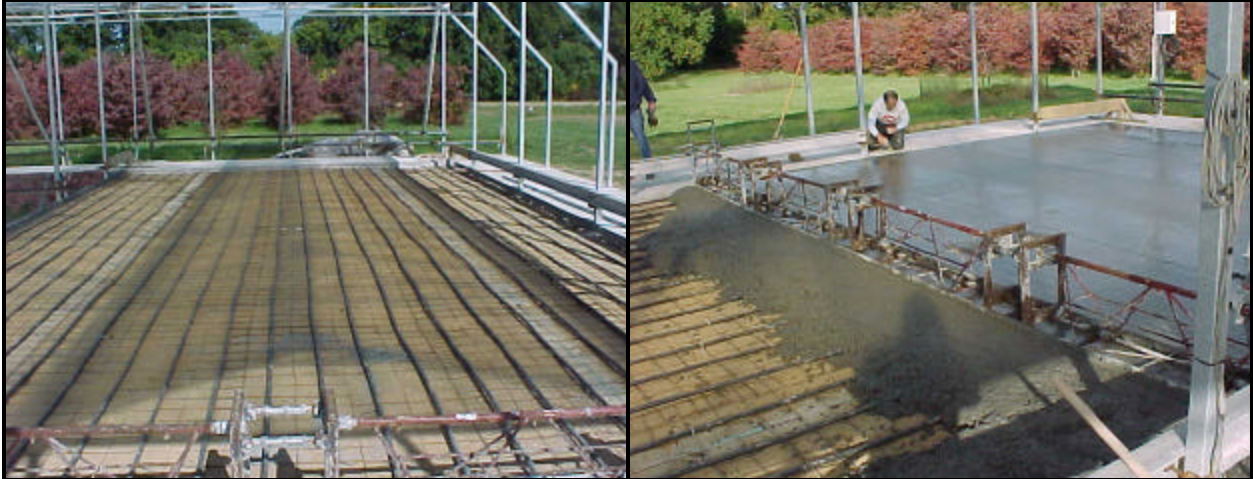
Photo 1. The (black) heating pipe is secured onto the reinforcing wire just prior to pouring the concrete. The pipes are spaced 12 inches on center.
