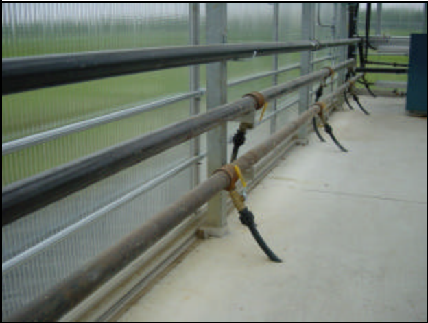
Photo 3. The plastic heating pipes are emerging from the concrete floor and are attached to the supply and return lines, which are connected to the hot-water boiler. Two valves are installed in each heating loop in case the loop needs to be isolated for maintenance or repairs.
