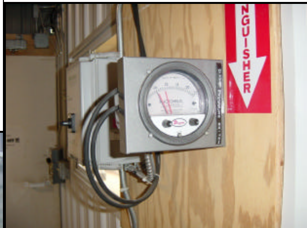
Photo 3. Differential pressure sensor and switch.
