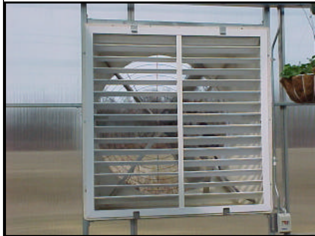
Photo 1. Ventilation fan with louvers.
