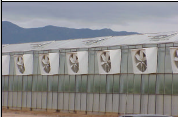
A view of the fans installed along the two side walls.
