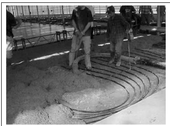
Three pictures of a heated concrete floor installation at John van Vugt near Pequannock, New Jersey.
